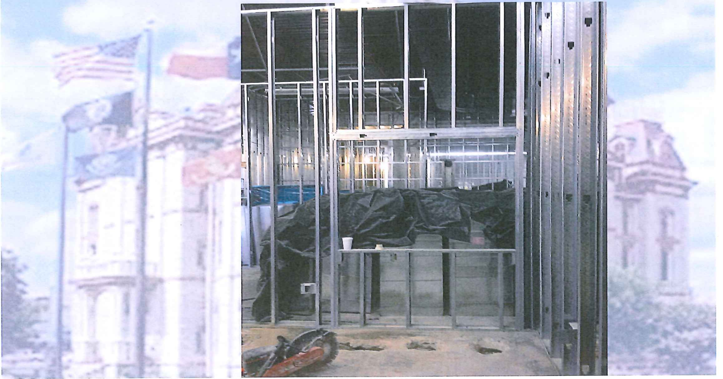
Tina's office next to I/T room looking into district clerks reception area
